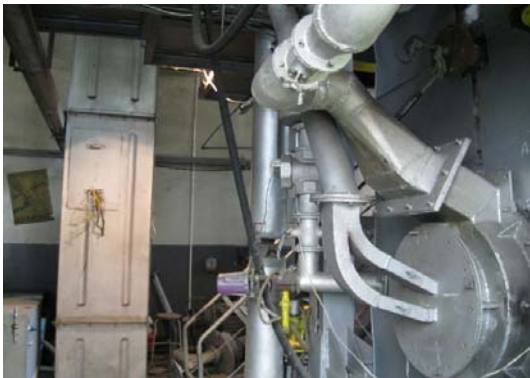
Figure 2. The embrasure of the UPB pilot boiler where the suspension sawdust burner was mounted
